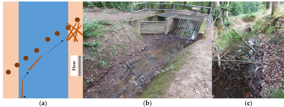
Figure 11. (a) Functioning of a deadwood lock as well as examples of typical stream locations within a forest where a deadwood lock would be suitable to protect a downstream screen from damage: (b) screen number 24; and (c) screen number 28.
